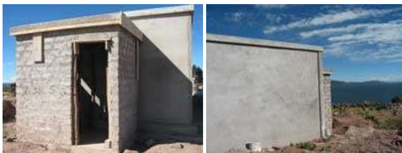
The concrete buildings built by the Huayllano artisans over a spring, ready for a pump and electric generator to be installed providing fresh water to their houses
